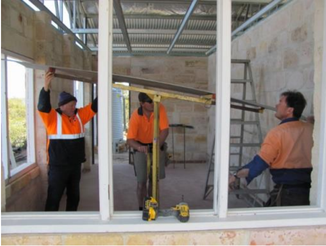
Ric Pepper, Kayne Hamilton and Chris Newton winding up a sheet of iron for the ceiling. Photo G.Craig.
